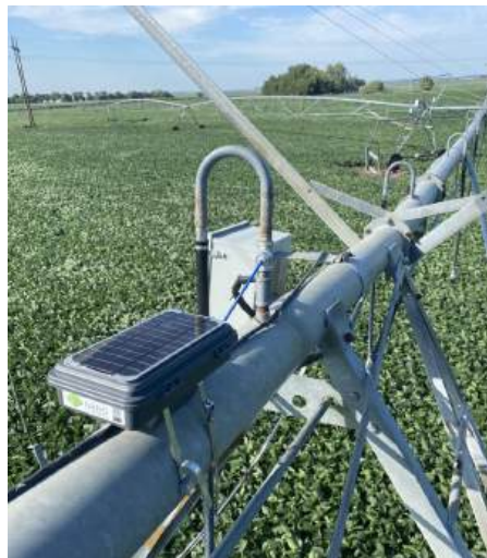
Nano Solor Installed
